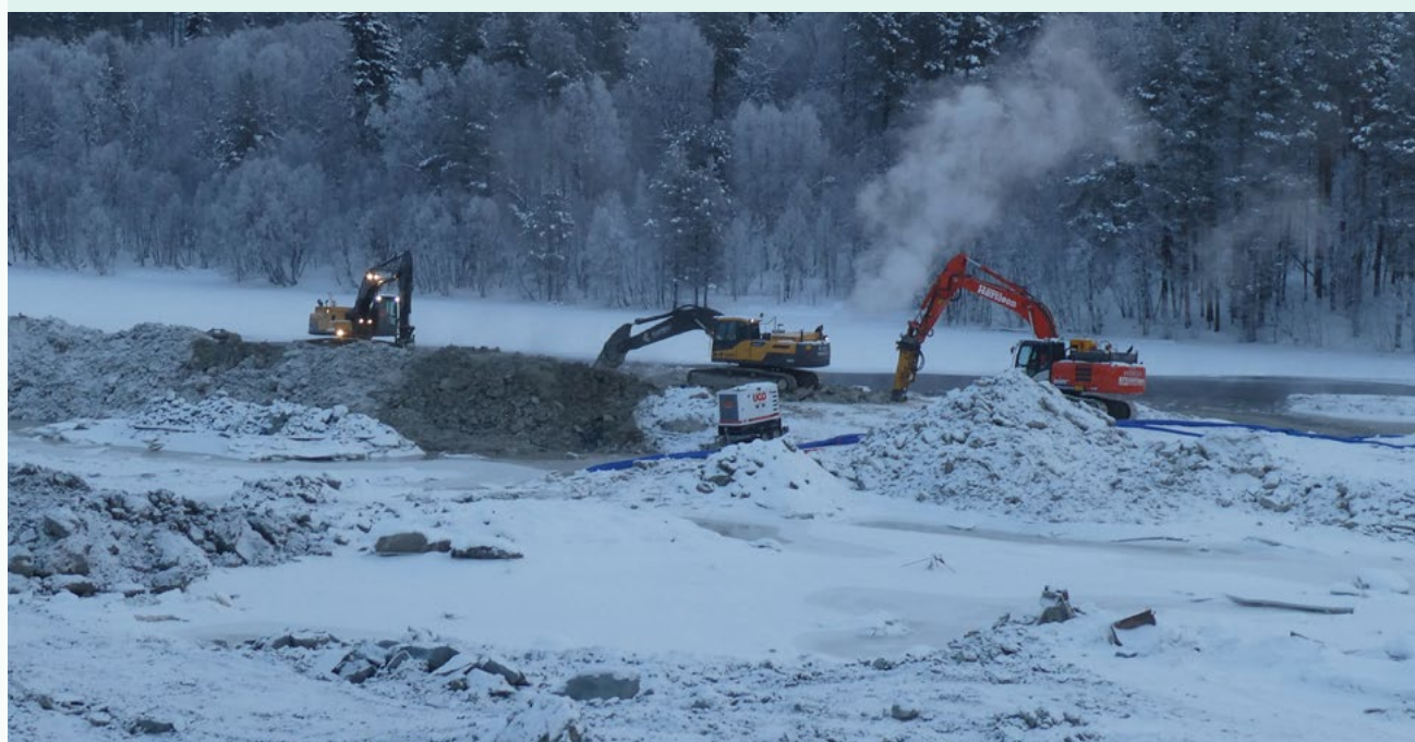
The local contractor HR Entreprenører is in the process of establishing a catchment area.
