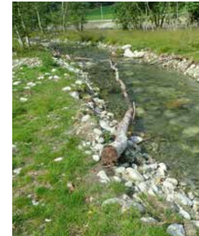
In the spring of 2020, a new side branch in the Aurlandselvi was built by Tokvam, and within a few months the vegetation along the side branch was well established. Photo: Bjørn Otto Dønnum
